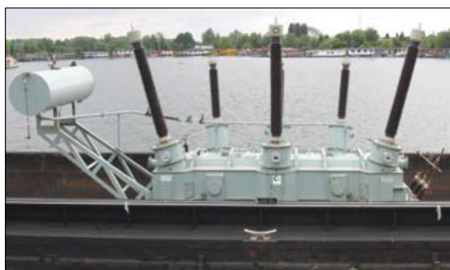
315 MVA, 440/220/133 kV Auto Transformer at KEMA, Netherlands
