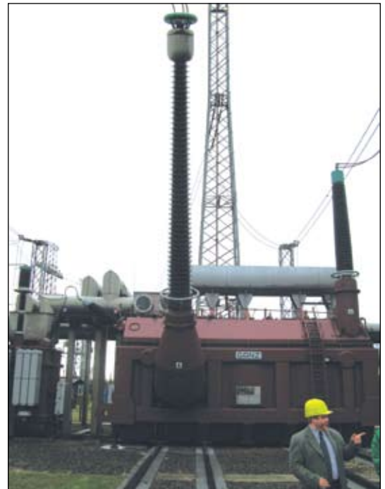
367 MVA, 750 kV Single Phase Auto Transformer, Albertissa, Hungary.
