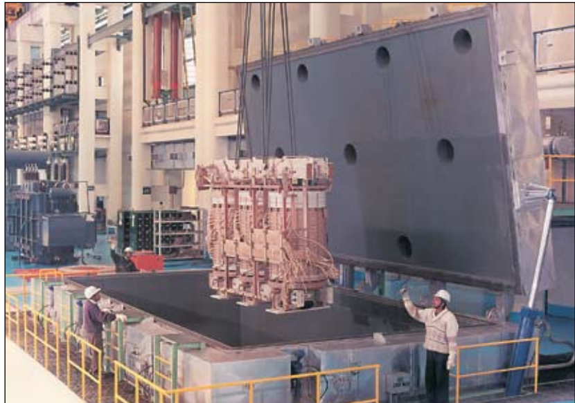
Micafil VPD Facility
