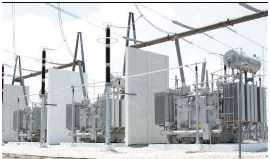
3 x 250, 550/275/33 kV, Single Phase Auto Transformer, Kapar Substation, TNB Malaysia
