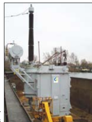
102 MVA, 400 kV Single Phase Generator Transformer at KEMA Netherlands
