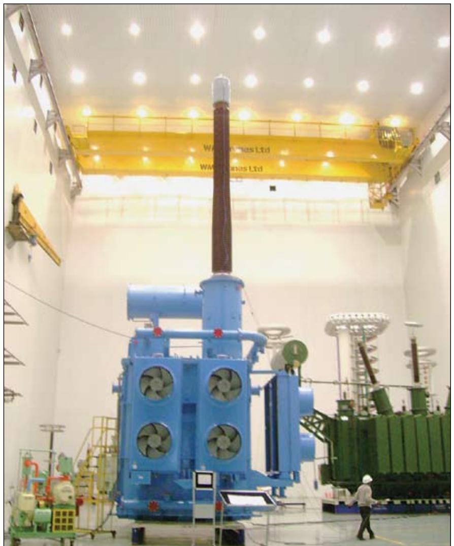
260 MVA, 765 kV Single Phase Generator Transformer supplied to NTPC Sipat
